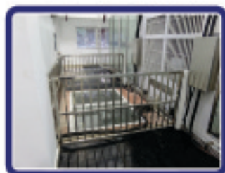
Cooling Water Return Pool
