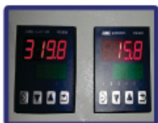
Temperature and Pressure Display on the Platform
